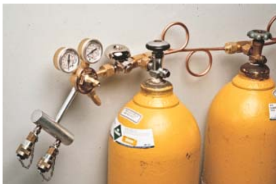
Air cylinders connected by tee blocks and pigtails, equipped with Audi-Larm Audible Alarm and air cylinder pressure regulator.
